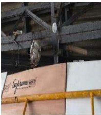
Flameproof light cable gland packing found damaged, need to repair/ replace immediately
