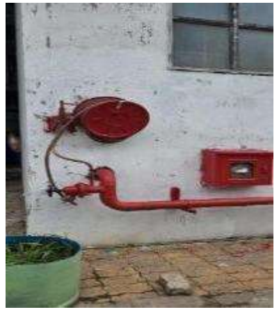
Hose reel drum found damage to be repaired & nozzle needs to be provided
