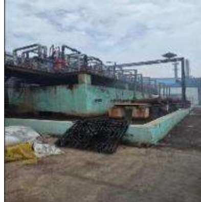
ETP needs to be maintained as per consent condition
