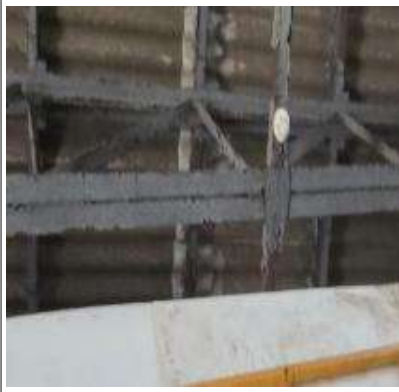
Structure found rusty needs to be painted
