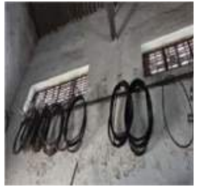
Crack & water seepages found on wall needs to repaired
