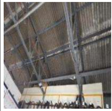
Flameproof electric fitting needs to be provided
