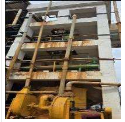
Structure found rusty needs to be painted
