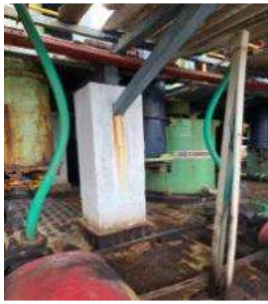
Crack found developed on the beam needs to be repaired & structure rusty to be painted, cladding sheet found damage needs to be repaired.
