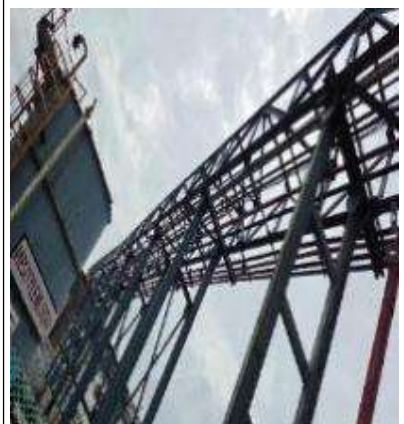
Pipe & cable support structure found passing over PESO license area, needs to be relocated away from storage tanks
