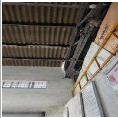
Water seepages found on wall needs to be repaired & Side cladding sheets found in damaged conditions needs to be replaced
