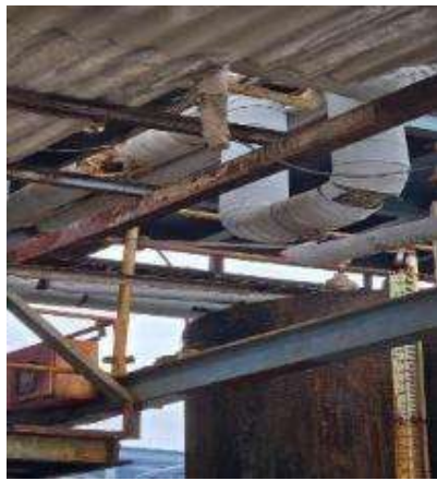
Sheet found damage needs to be repaired & structure found rusty need to be painted
