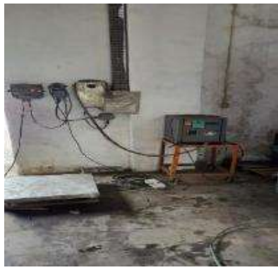
Oil found on the floor need to be clean & Loose cables arrange properly
