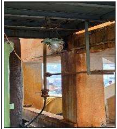
Structure rusty needs to be painted
